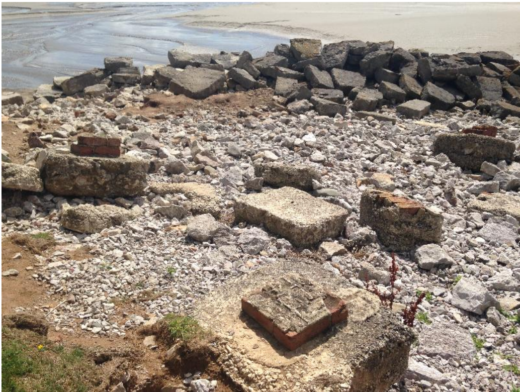
Plate 12. Brick and concrete remains, forming part of a structure constructed above the embankment (Site 1A). Note, the collapsed rubble/remains of the quay/jetty in the background (Site 1B).
