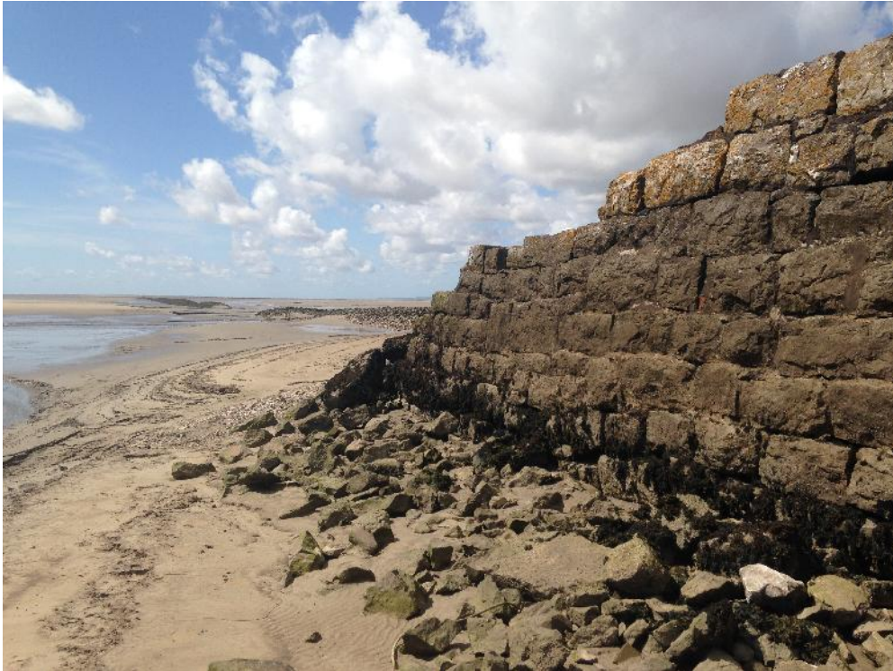
Plate 10. The south-western limits of the stone quay/jetty with the embankment (Site 1A) in the background (August 2014)
